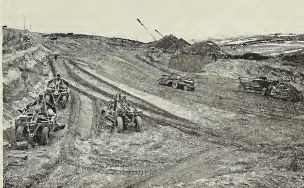
Sand is hauled by truck from big pits to build foundations for the runways and dispersal areas.
